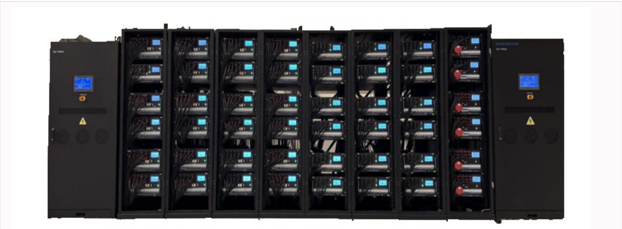
◆ Load bank hall, installed Multi-rack array under commissioning
